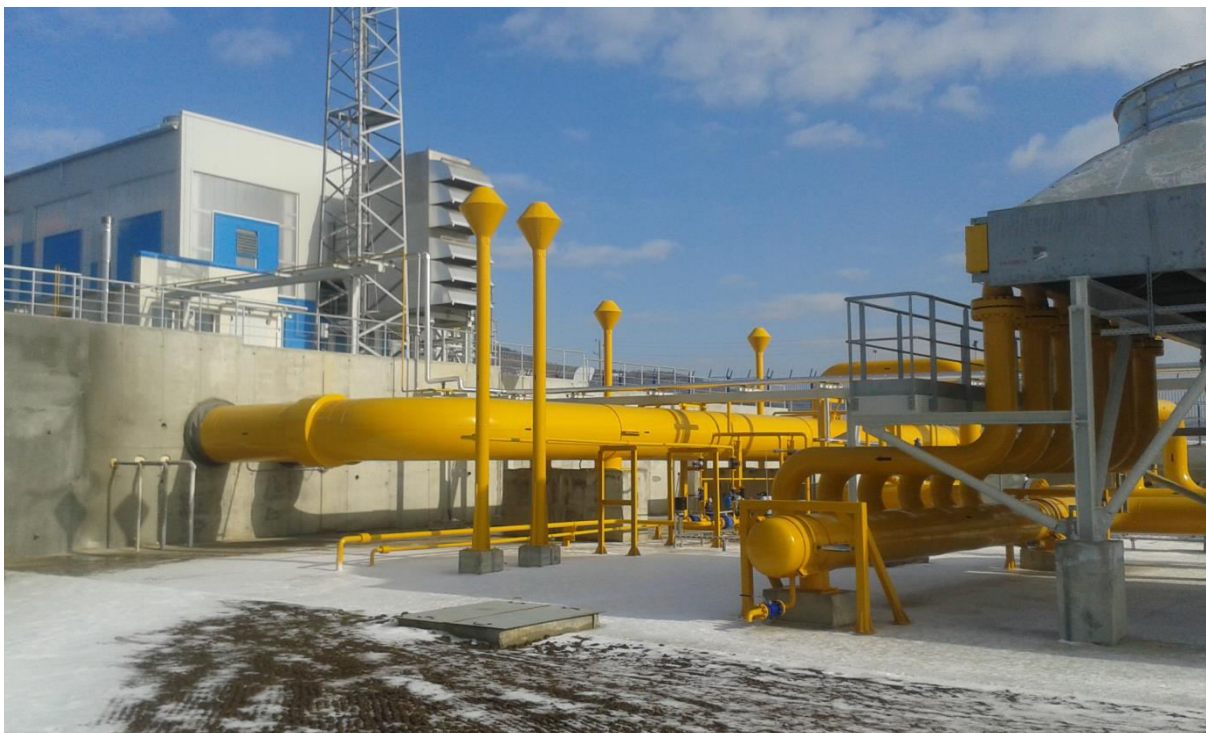
Compressor Station Lozenets
