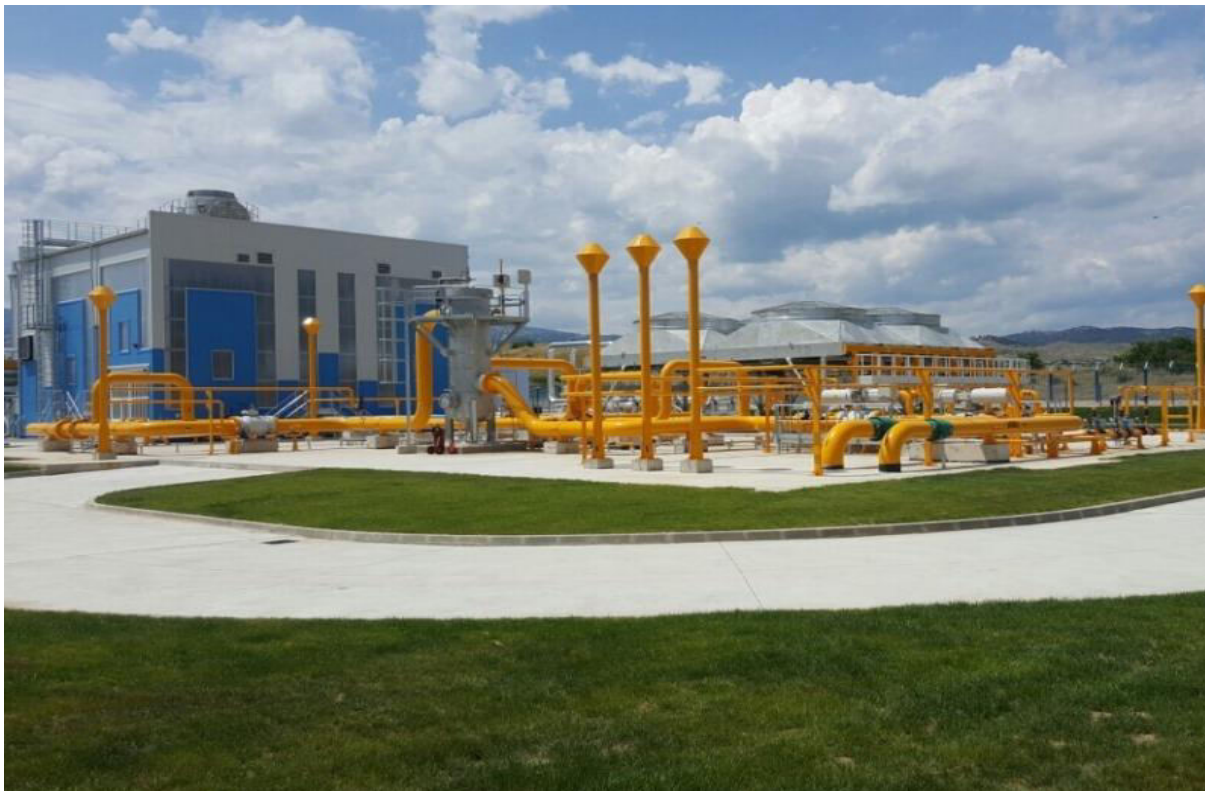
Compressor Station Ihtiman
