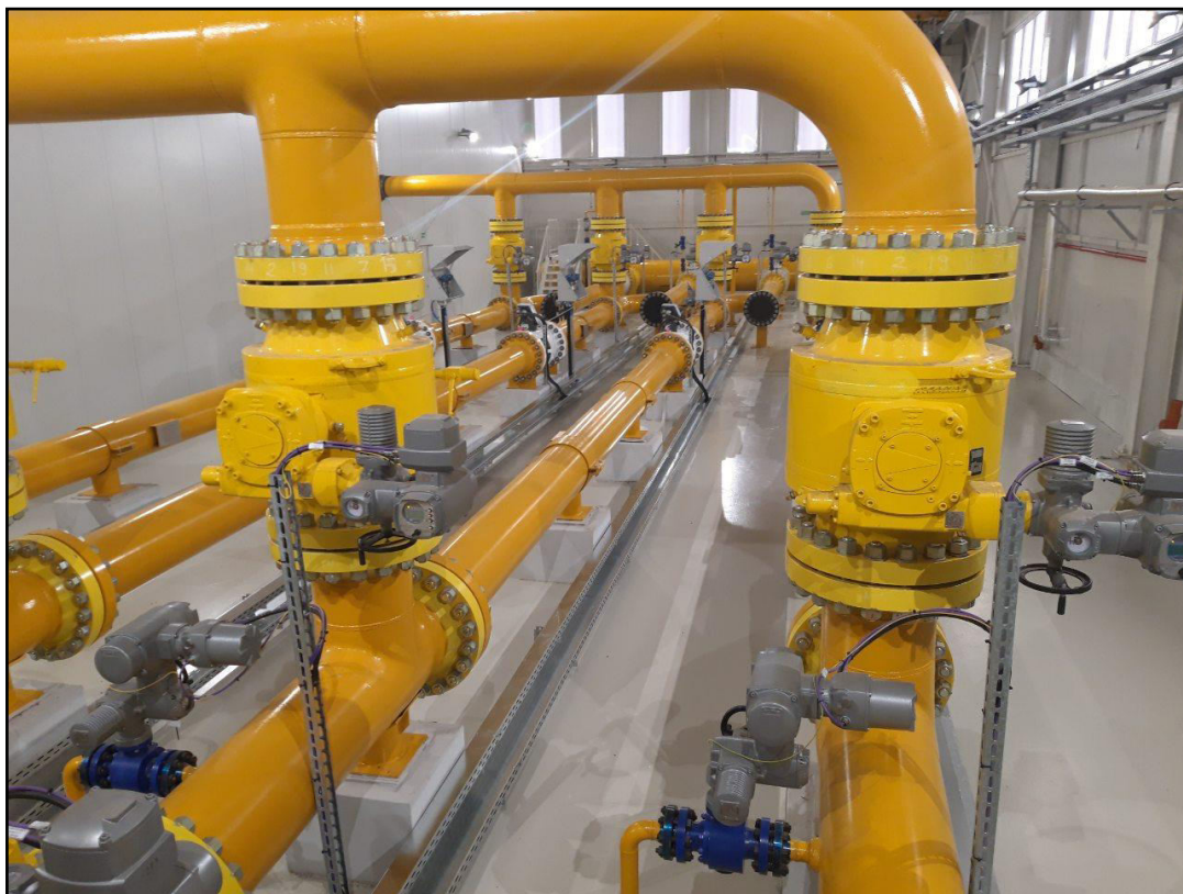
Metering lines in GMS
