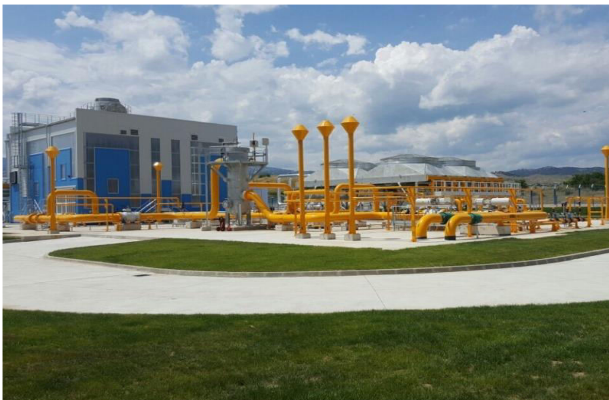
Compressor Station Ihtiman
